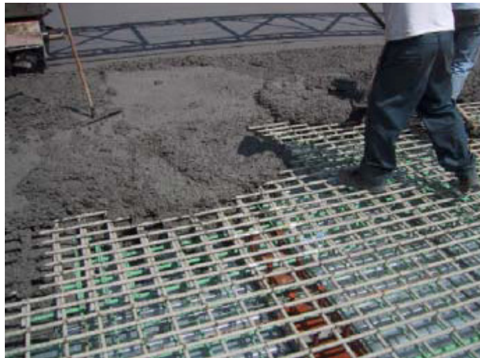
Placing concrete in a bridge slab reinforced with glass FRP bars (top layer) and epoxy coated steel bars (bottom layer)
